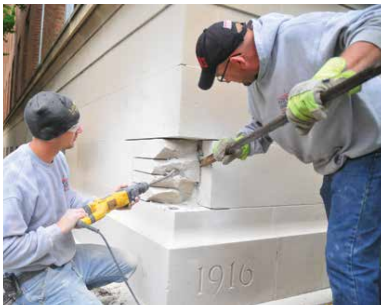
Krivda and Son Masonry employees (from left) Ben Krivda and Chris Krivda begin the process to remove the Avery Hall cornerstone on May 12, 2014.
